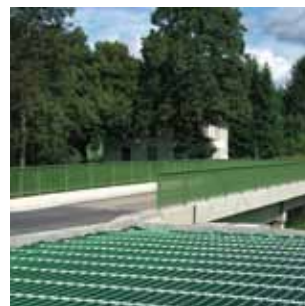
Open space heating
