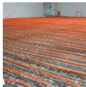
Industrial floor heating
