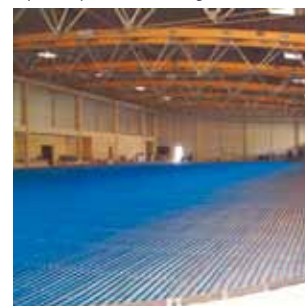
Chilled area, ice stadium
